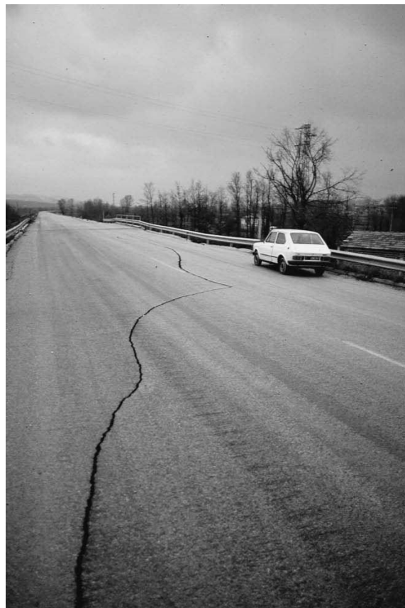
Fig. 4. Surface cracking on a road embankment after the 1980 Irpinia earthquake, Lioni, Italy.
