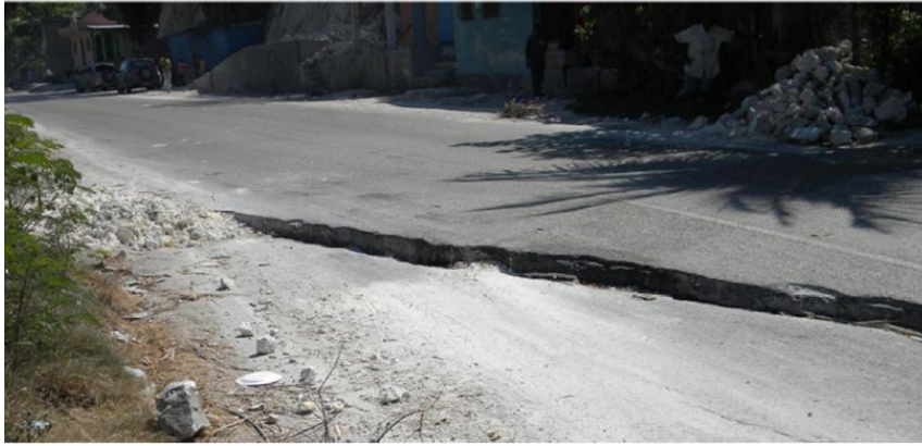
Fig. 2. Vertical cracking observed along road alignments following the Haiti earthquake.
