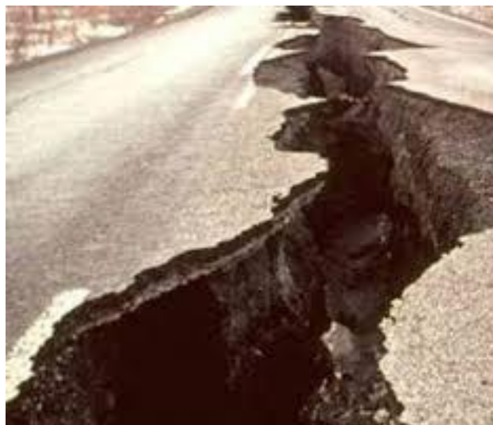
Fig. 7. Longitudinal cracking in a road embankment during the Peru earthquake, reflecting tensile stresses along the road axis.
