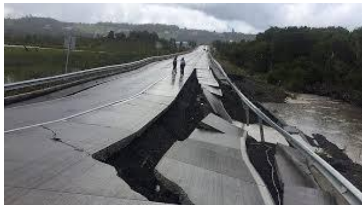
Fig. 6. Shear failure in a road embankment during the 2010 Chile earthquake, showing notable lateral pavement displacement.
